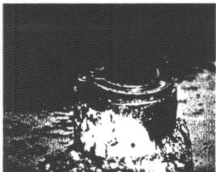
Fig. 1. The twin-nozzle abrasive jet cutter's primary advantage was its remote positioning and operating capabilities. This allowed wellhead equipment to be severed from burning wells and precluded the need for personnel to enter oil-flooded cellars (top photo). After cuts were made, wells were killed using stingers or capped using several different types of capping assemblies. Lower photo shows flow out of 7-in. casing that is being restricted by tubing, which fell downhole after being cut.
